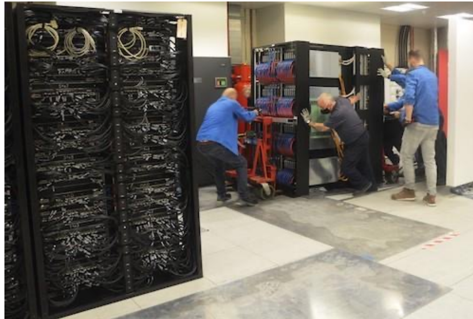
Installation of the UK Supercomputer “Archer2” 750,000 compute cores
